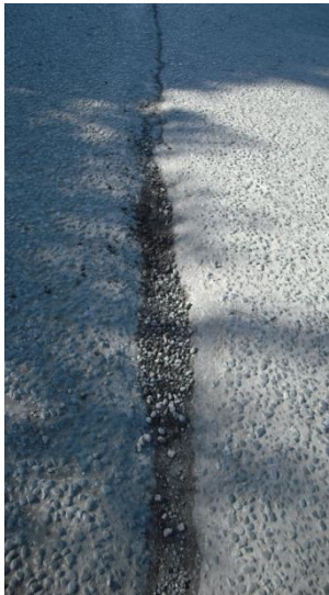
Typical joint failure
