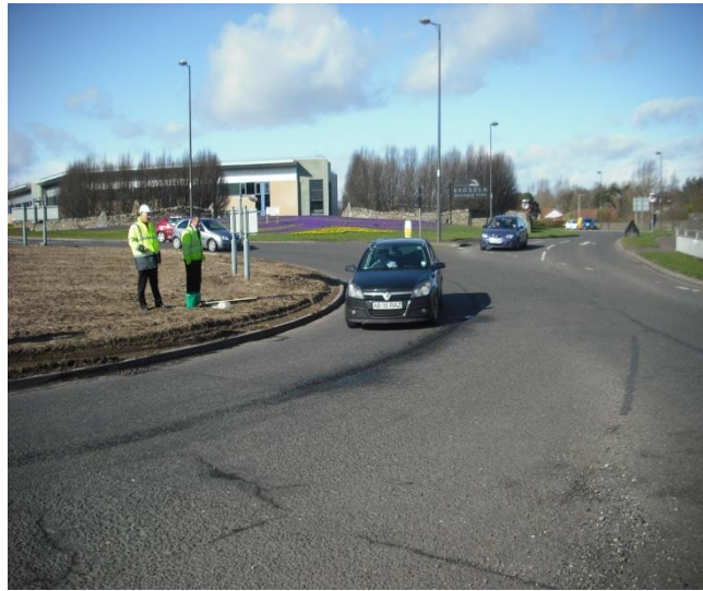
Viafix tipped into wet defect, compacted to finish by traffic. Time in carriageway <2 minutes (12 th Feb 2009)
